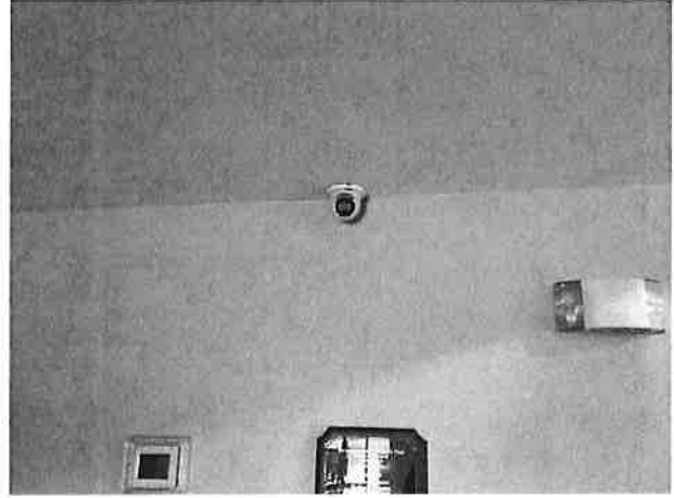
Security system camera
